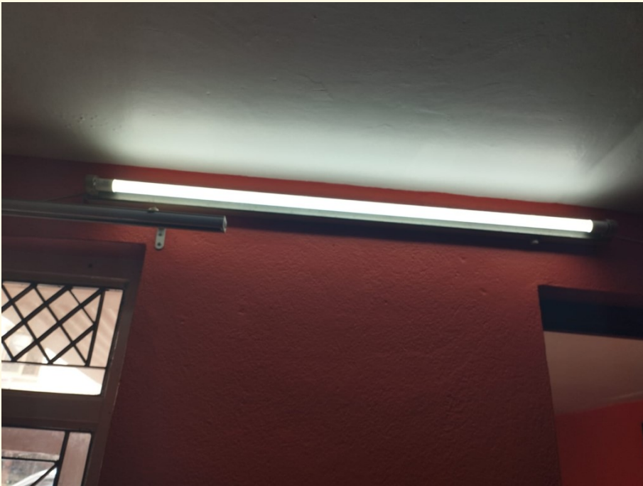
Energy saving LED lights
